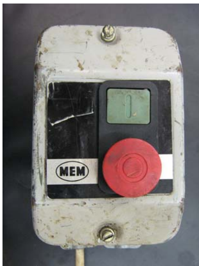
Figure 10 A typical older DOL starter
